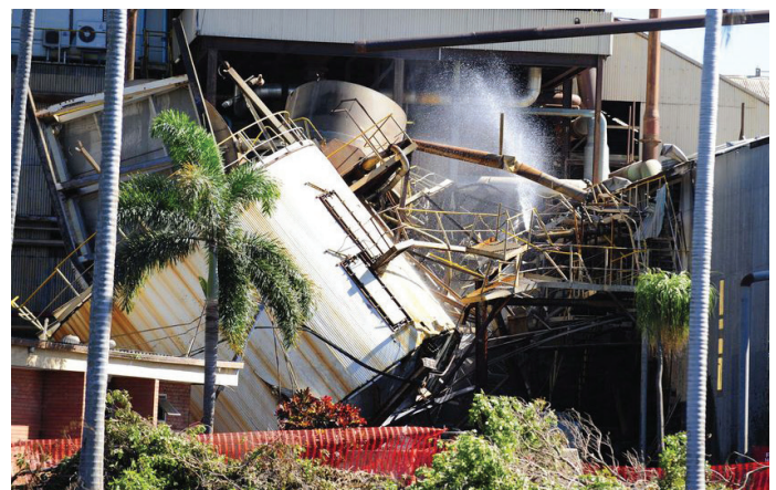
This sugar mill collapsed due to advanced corrosion. Long-term corrosion protection is only possible with optimum surface preparation.
