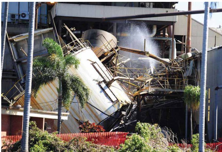
THIS SUGAR MILL COLLAPSED DUE TO ADVANCED CORROSION
